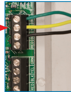
Figure 12. Jandy Pro Series VSP Connection to Pump
