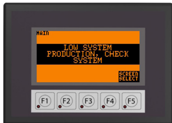
Example with Fault Message (Flashing Amber Backlight)
