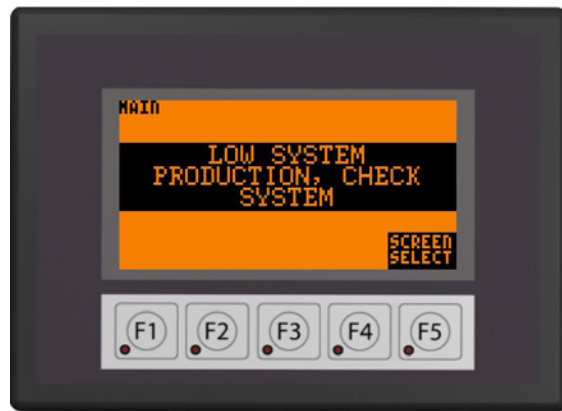
Example with Fault Message (Flashing Amber Backlight)
